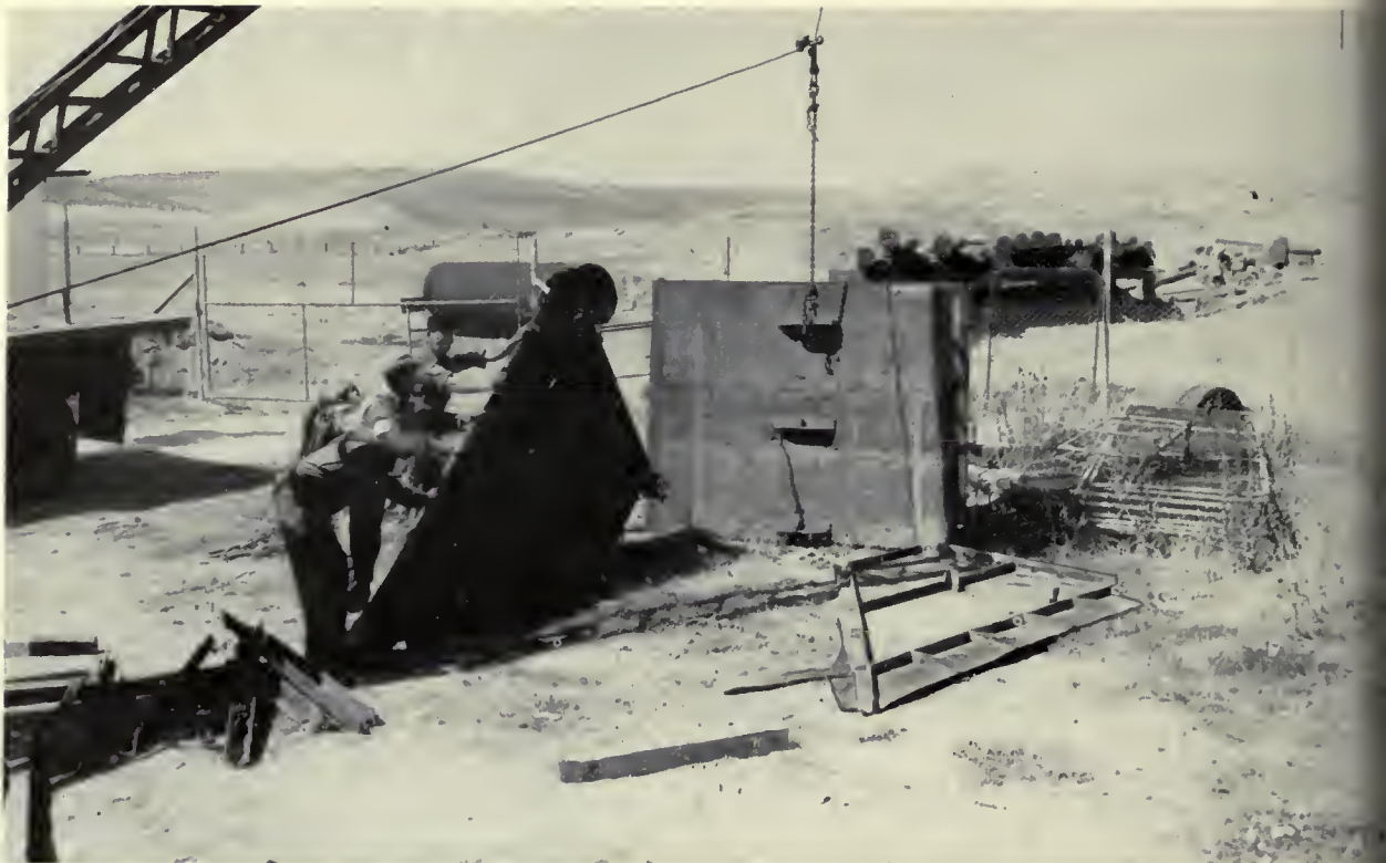
EASY TO ASSEMBLE. —A Contra Costa maintenance crew assembles the newly developed cofferdam in a short time, to meet an emergency.
